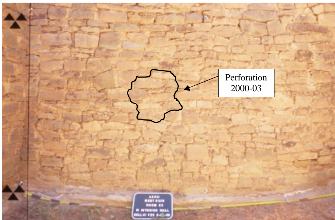
Figure 03A. West interior wall of Room 63, looking southwest at location of wall perforation that was removed during FY-00 backfilling project. Pre-backfill photo taken June 24, 1999.
