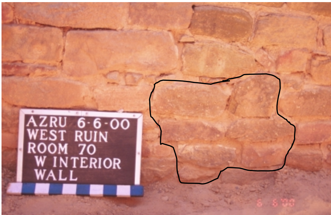
Figure 01B. West interior wall of Room 70, looking southwest, prior to removal of Perforation 2000-01 on June 6, 2000. Perforation is outlined.
