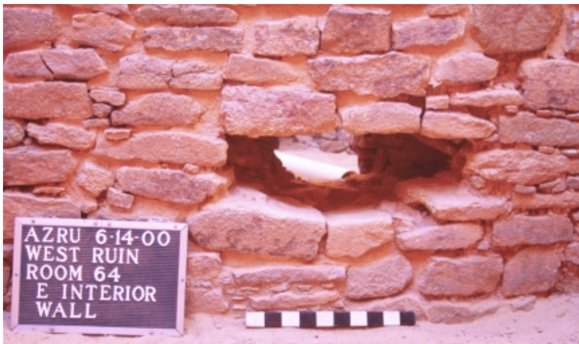
Figure 03F. East interior wall of Room 64, looking northeast, after initial wall penetration on June 14, 2000.
