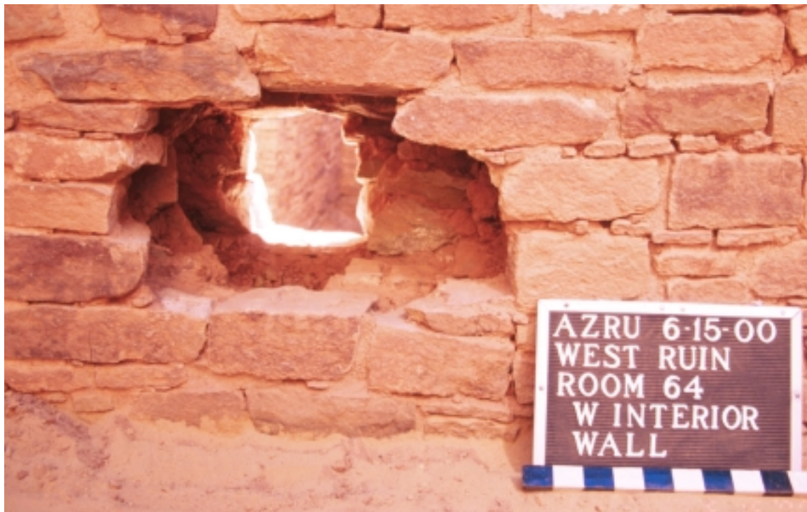
Figure 04B. West interior wall of Room 64, looking southwest, after initial wall penetration. The stone in center below the initial perforation was later removed to accommodate pipe.
