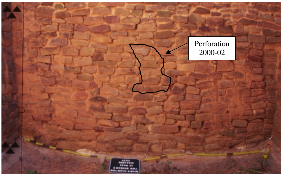
Figure 02E. East interior wall of Room 63, looking northeast at location of wall perforation that was opened during FY-2000 backfilling project. Pre-backfill photo taken June 24, 1999.
