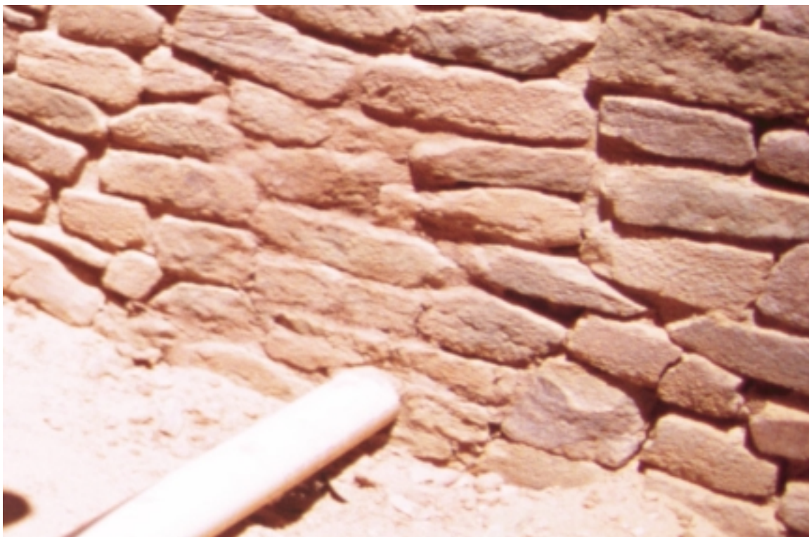
Figure 02H. East interior wall of Room 63, looking north, after masonry closure around Perforation 2000-02.
