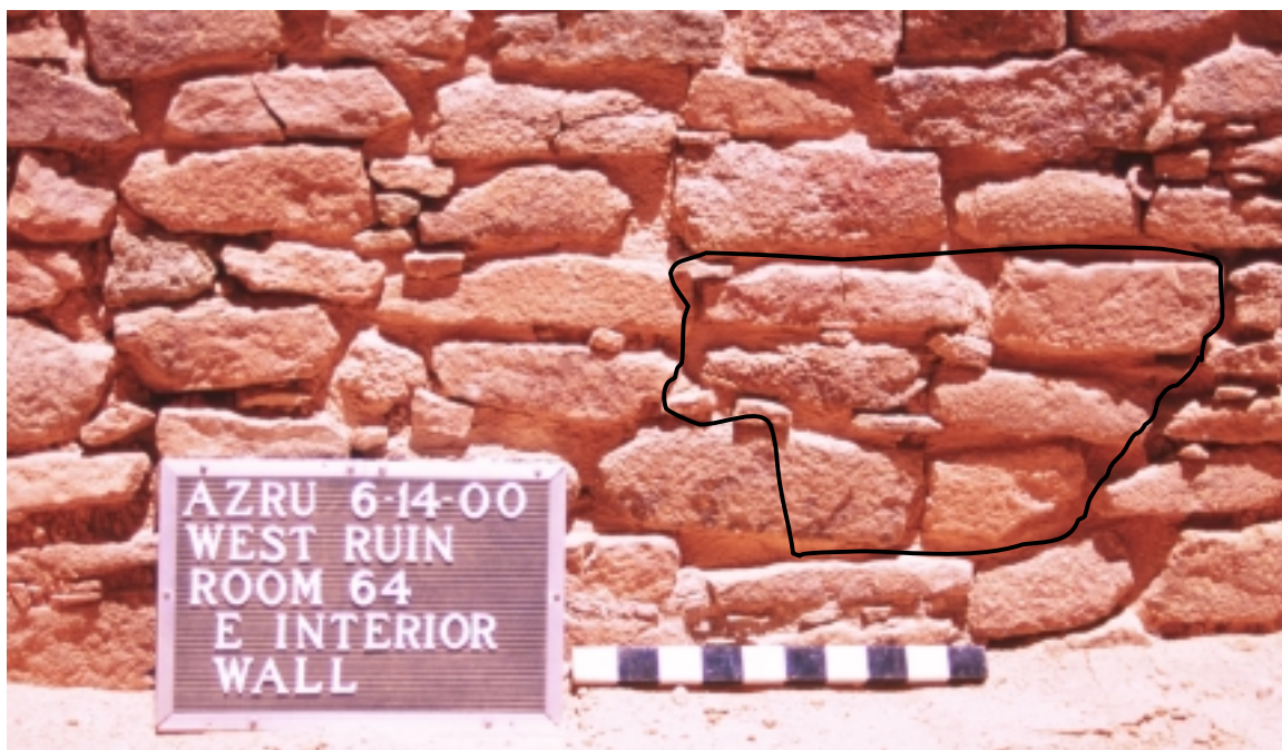
Figure 03E. East interior wall of Room 64, looking northeast, prior to removal of Perforation 2000-03 on June 14, 2000. Perforation is outlined.
