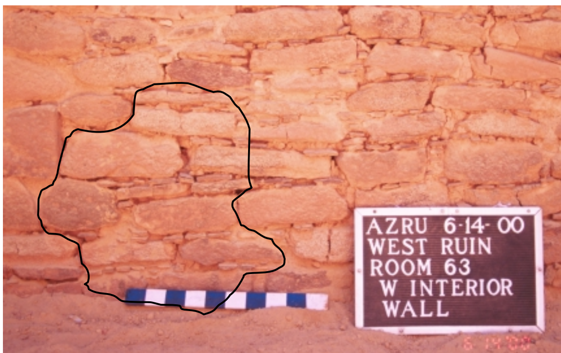
Figure 03B. West interior wall of Room 63, looking southwest, prior to removal of Perforation 2000-03 on June 14, 2000. Perforation is outlined.
