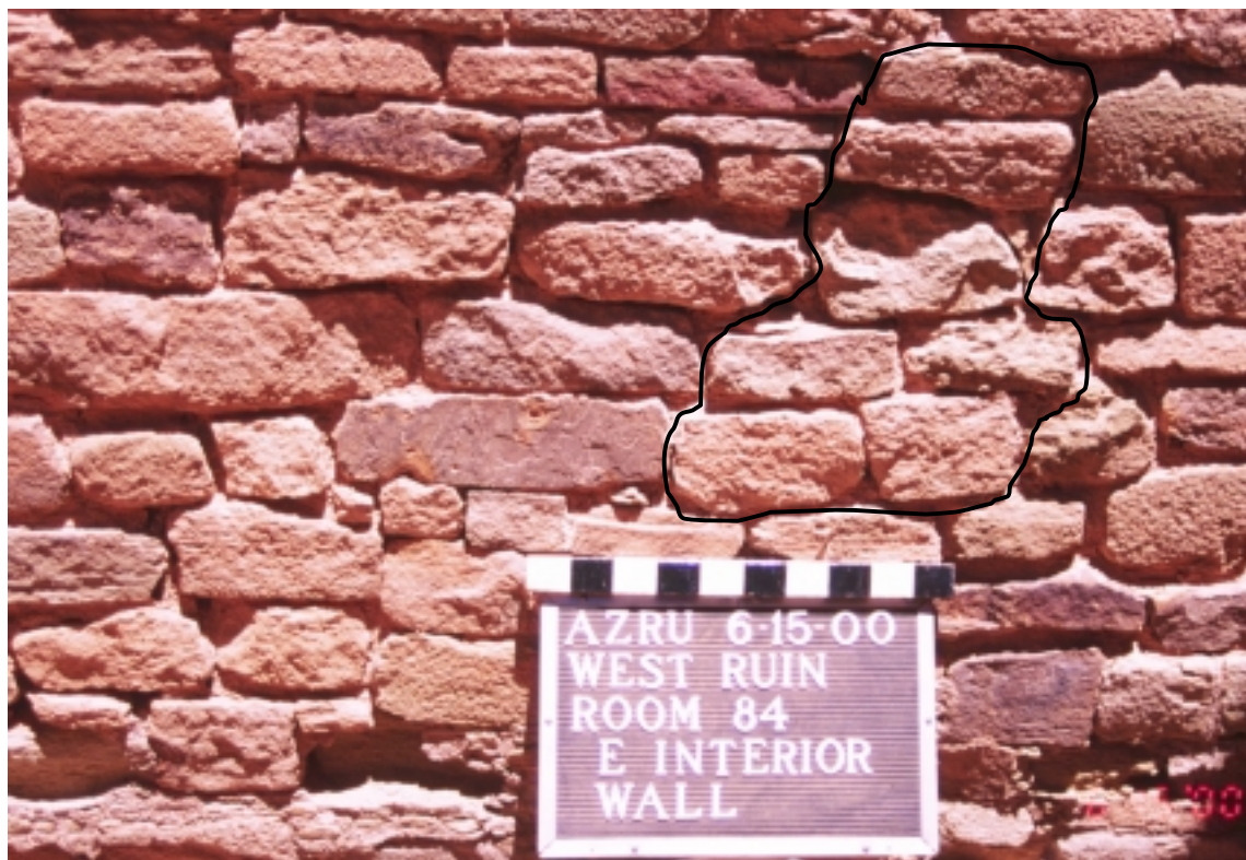
Figure 04F. East interior wall of Room 84, looking northeast, prior to removal of Perforation 2000-04 on June 15, 2000. Perforation is outlined.
