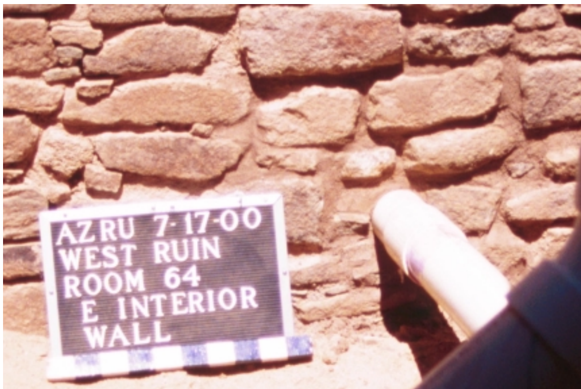
Figure 03G. East interior wall of Room 64, looking NE, after masonry closure around Perforation 2000-03.
