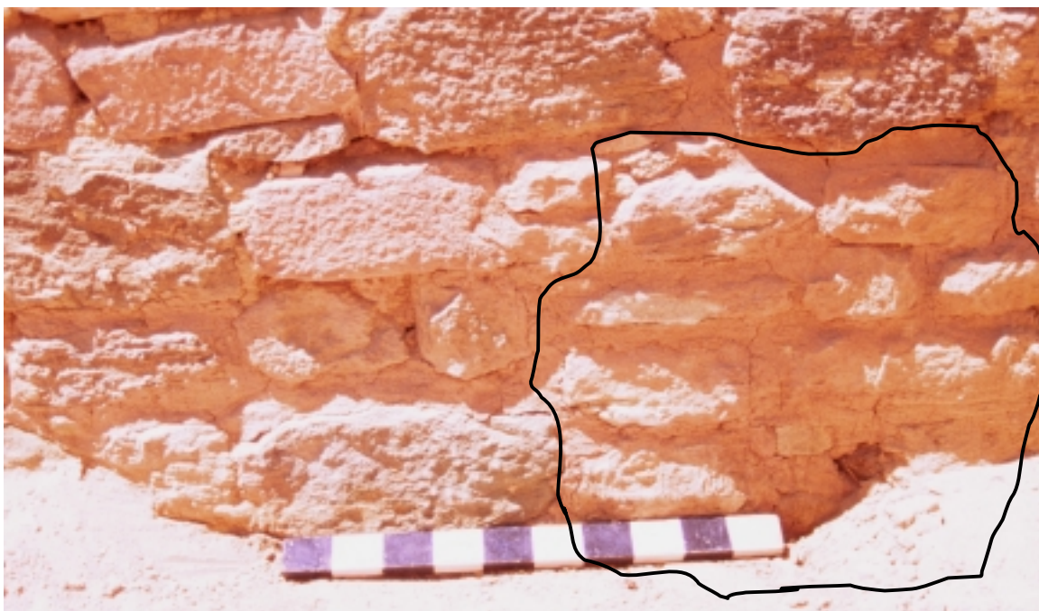
Figure 05B. East exterior wall of Room 70, looking southwest, prior to removal of Perforation 2000-05 on June 20, 2000. Perforation is outlined.
