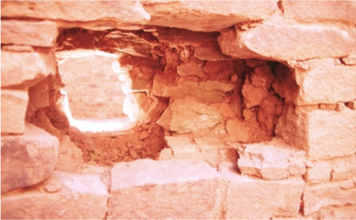
Figure 04C. Perforation 2000-04 through west interior wall of Room 64, looking west, showing semi-coursed masonry in solid core construction.
