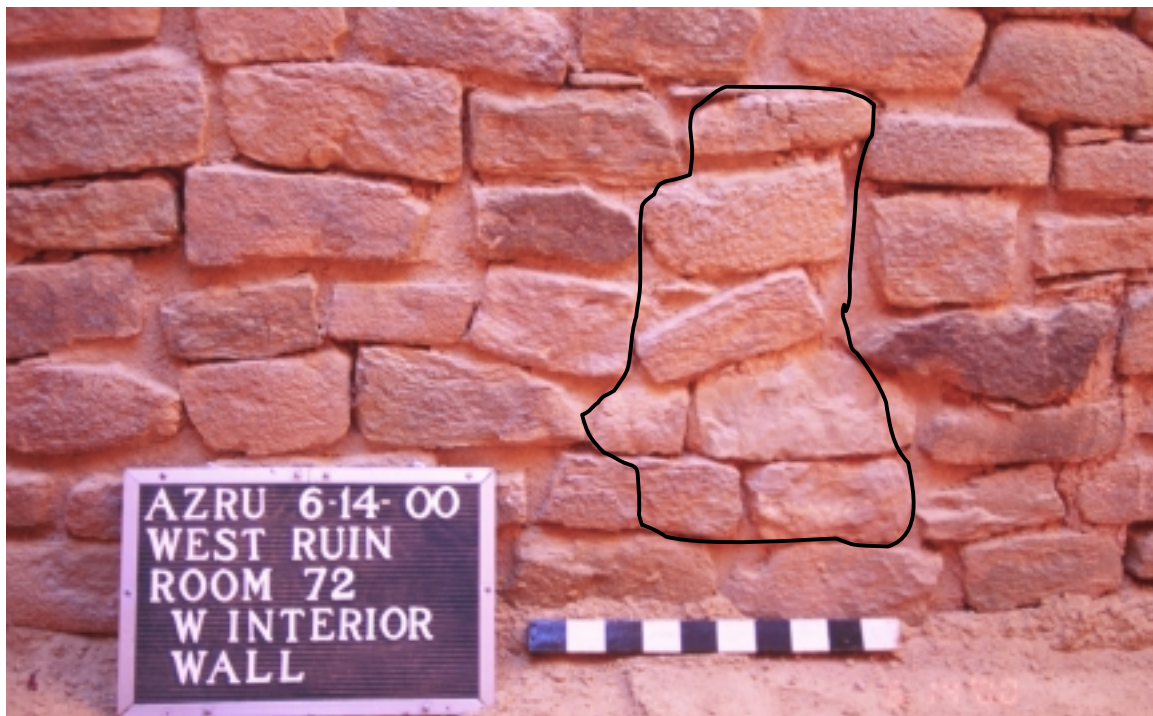
Figure 02B. West interior wall of Room 72, looking southwest, prior to removal of Perforation 2000-02 on June 14, 2000. Perforation is outlined.
