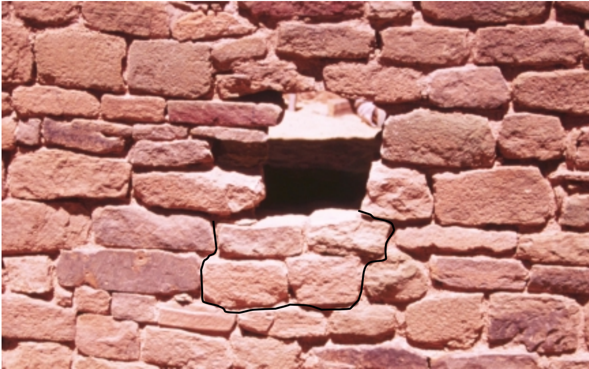
Figure 04G. East interior wall of Room 84, looking northeast after initial wall penetration. Area that was later enlarged to lower drainage pipe is outlined below initial perforation.
