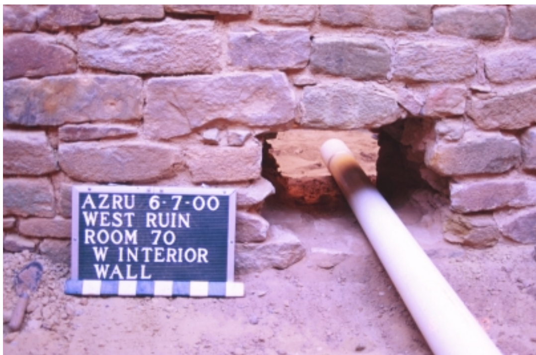
Figure 01C. West interior wall of Room 70, looking southwest, after initial wall penetration on June 7, 2001, showing initial placement of PVC pipe.
