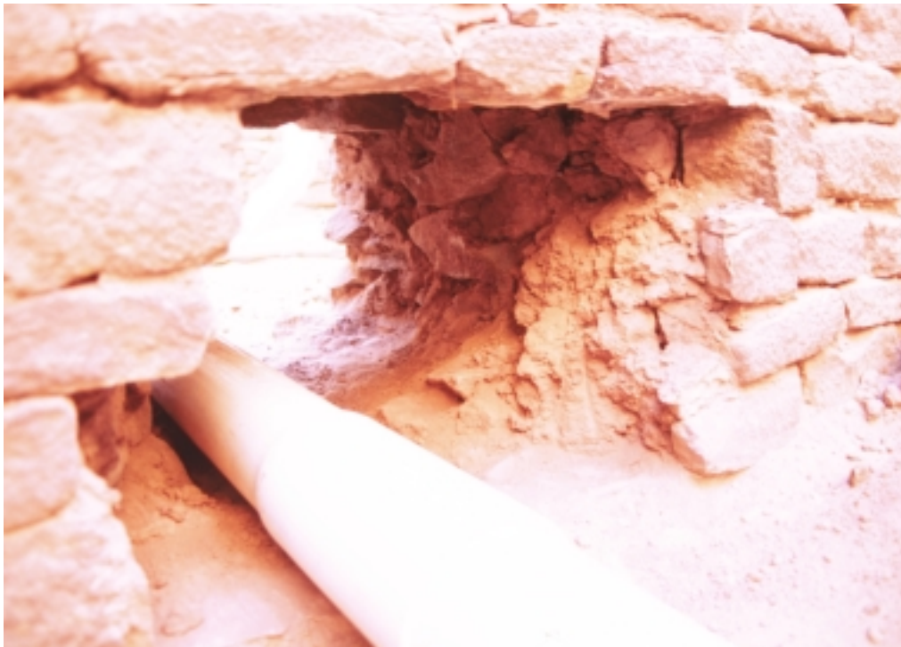
Figure 01I. Masonry-filled core construction in Perforation 2000-01, looking east from Room 71, after completion of penetration and installation of PVC drain pipe.
