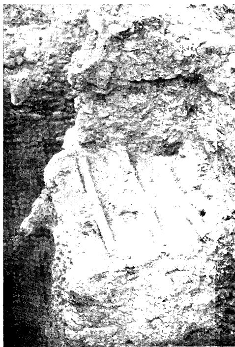
b. The Same Piece of Roof After the Removal of the Upper Portion of the Column. The cross members of the roof are plainly visible.
