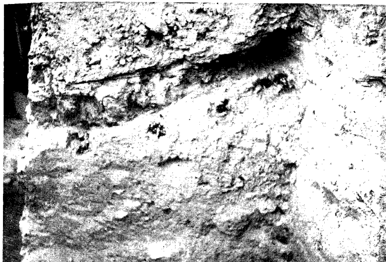
a. The Stratigraphy Column in Room 4 Which Contained a Section of the Original Roof.
